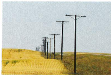
Three-phase power line
