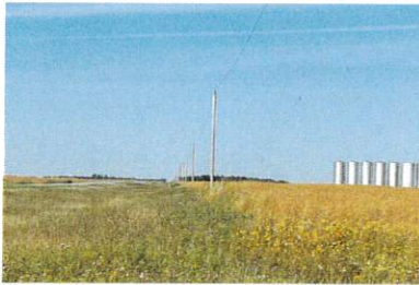
Single-phase power line
